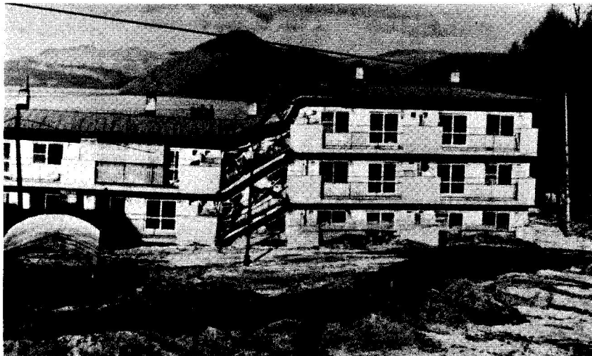
FIG. 2. BUILDING RUPTURED BY TECTONIC DISPLACEMENT, LAKE TOYA, JAPAN.
