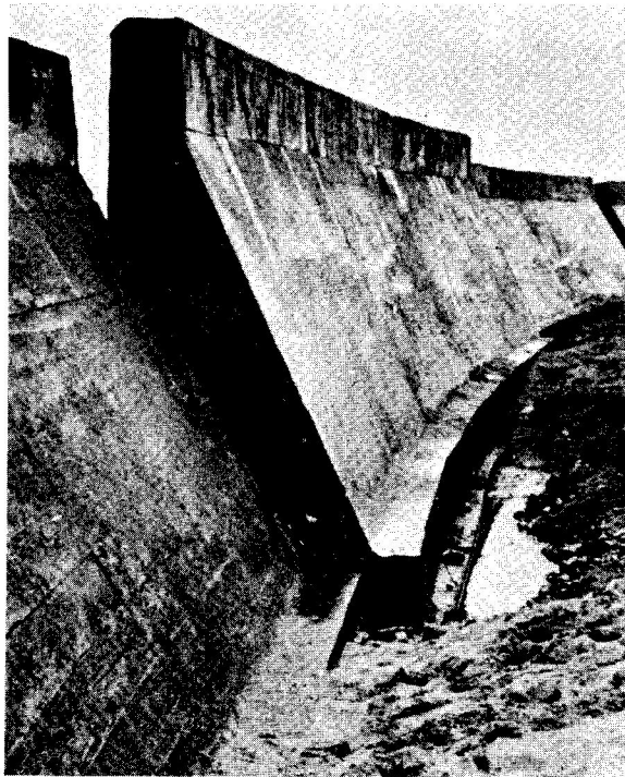
FIG. 10. GRAVITY RETAINING WALL DISPLACED BY LIQUEFIED BACKFILL (AFTER H. KAMASUMI, 1968).
