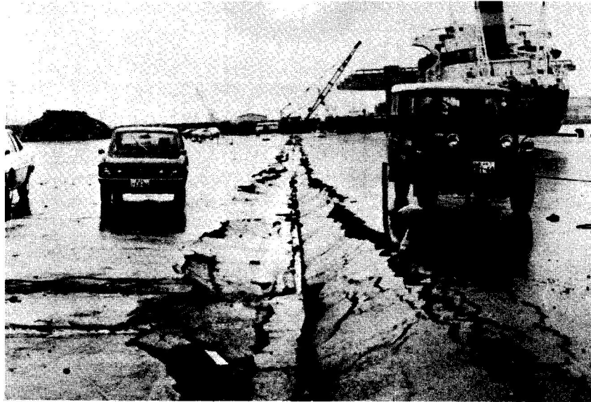
FIG. 9. SURFACE INDICATIONS OF MOVING BURIED ANCHOR WALL.
